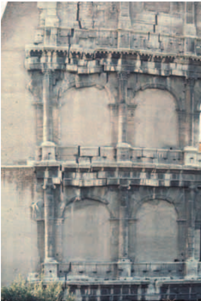
Figure 92. The Colosseum. The brick buttress built to support the east wall; a detail
