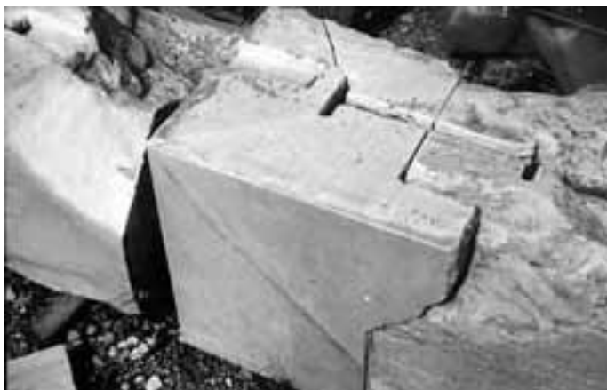
Figure 133. The Erechtheion: a block of marble restored by Balanos. The original stone has been cut in order to accommodate new marble. Iron cramps have since caused cracking of the original stone
