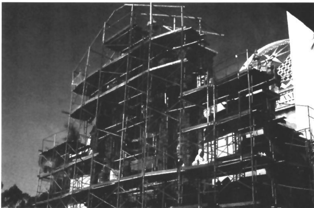
Figure 19. Scaffold for the restoration of the California Building. 1975. (Courtesy of K. L. Gauri).
