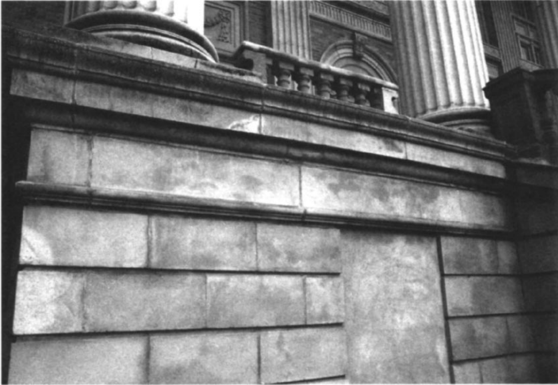
Figure 6. Exterior of Crescent Hill Baptist Church, Louisville, Kentucky, treated with epoxy resin in 1983. Figure shows the tones of the treated surface in 1989.
