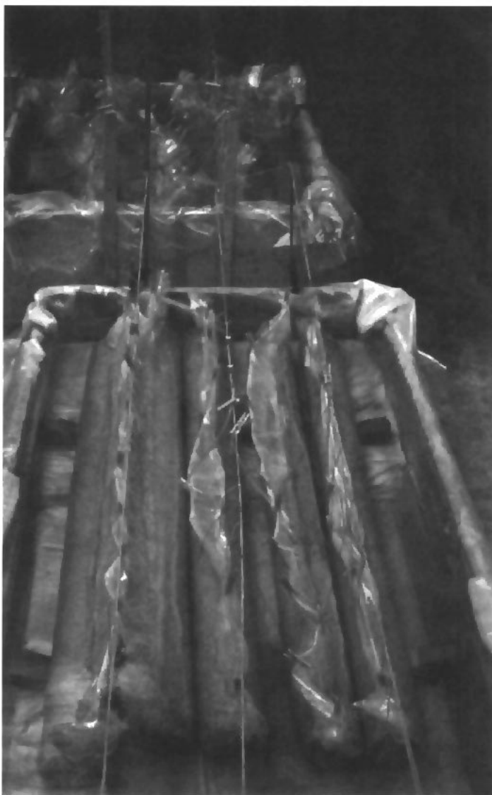
Figure 25. Twin columns of the Basilica of Santa Andrea in plastic containment in wood boxes (Lazzarini 1991).
