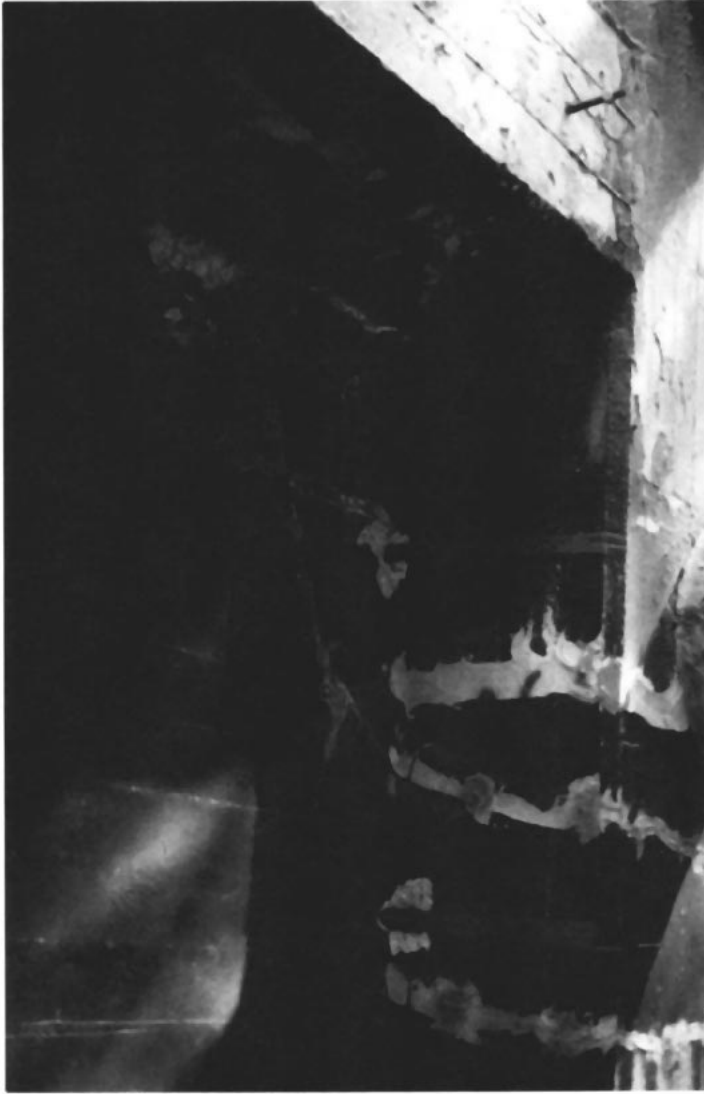
Figure 1. Epoxy repairs at Pier 187, Port of Los Angeles, thirty-six years after application. 1989.
